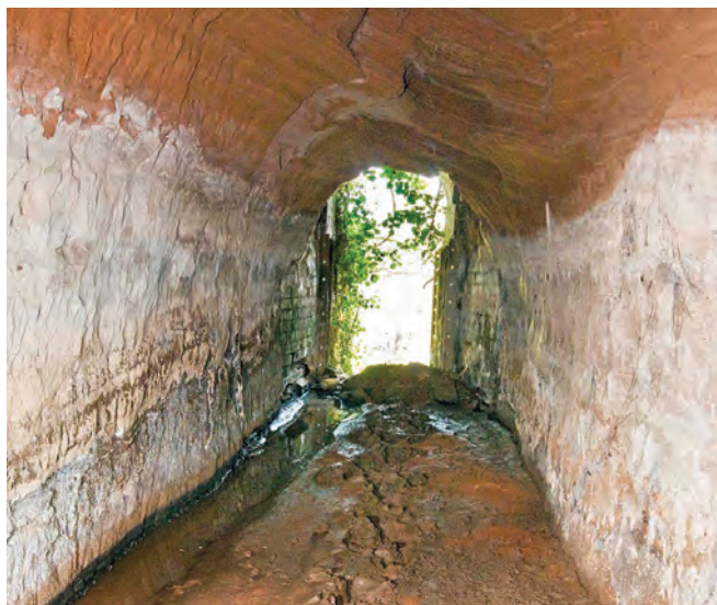
View along the tunnel leading to the waterwheel penstock. Note: the white marks indicating the historic water level, the muddy floor, and roof voids due to the spalling of the sandstone
